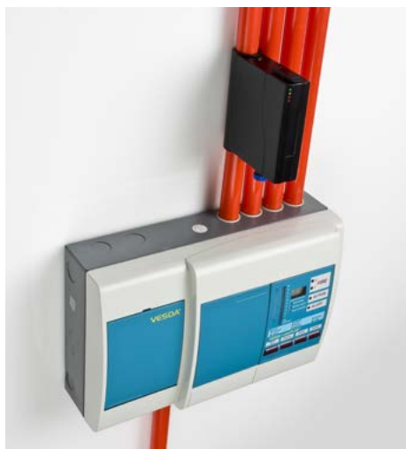
VESDA ECO installed on sampling pipe
