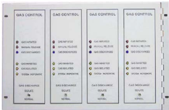
ME0441 4 Zone Gas Flood 7U Door
