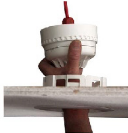
Pull the detector and back box assembly through the cutout into position on the ceiling tile
