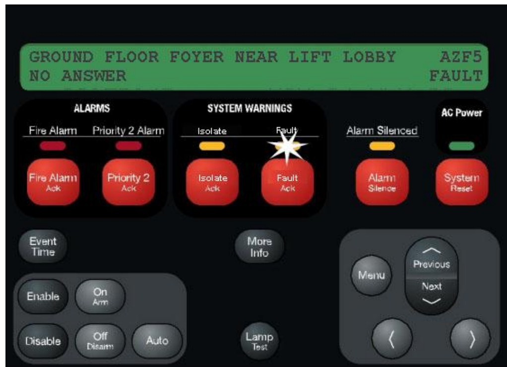
Figure 3-1. Operator Interface Showing Fault Condition
