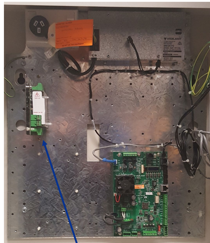
FP1117 Switching Module mounted in Grade 2 EWS
