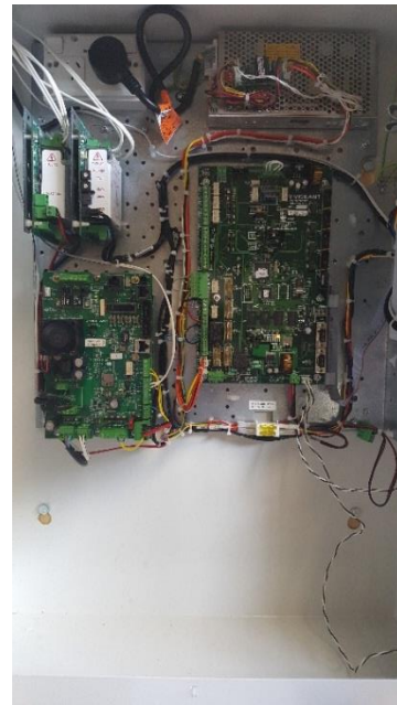
15U Gearplate with T-Gen2 & Splitter/Switching Modules
