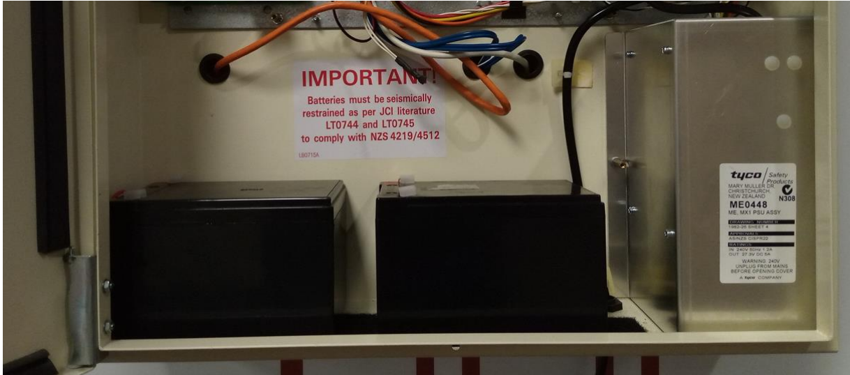
Figure 3.1 – Battery Restraint Label Fitted Inside an MX1 Slimline Panel
