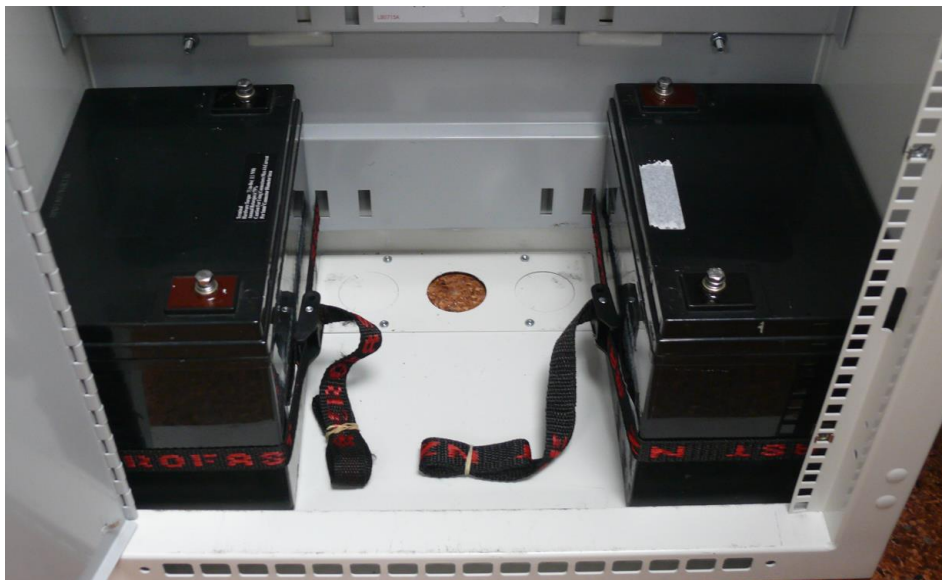
Figure 2 – Pair Of Restrained 75Ahr Batteries
