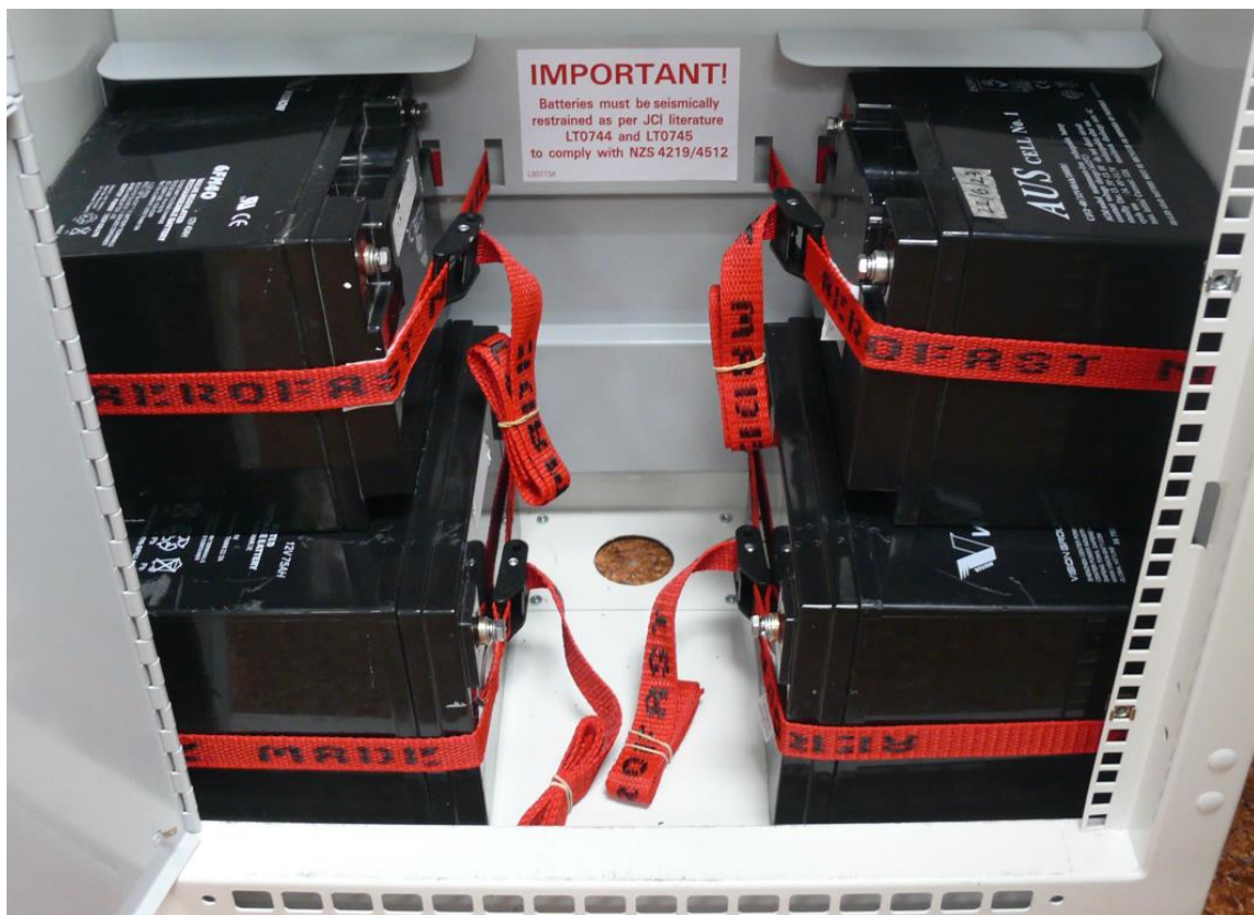
Figure 5 – Set Of Stacked Restrained Batteries two 40Ahr (top) and two 75Ahr (bottom) shown
